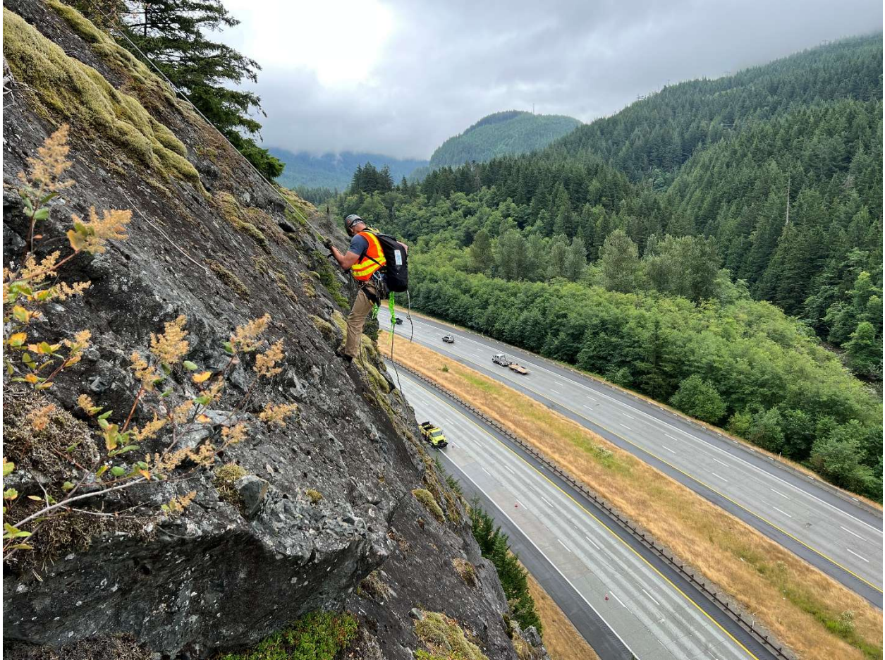
Exhibit 1. Engineering Geologist conducting slope assessment work on I-90, near North Bend, WA.
