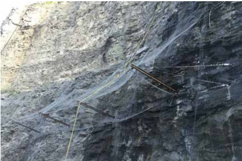
Figure 2. Temporary rockfall canopy above tunnel portal, Atlanta, GA. (Photo by Scarptec, Inc.)
