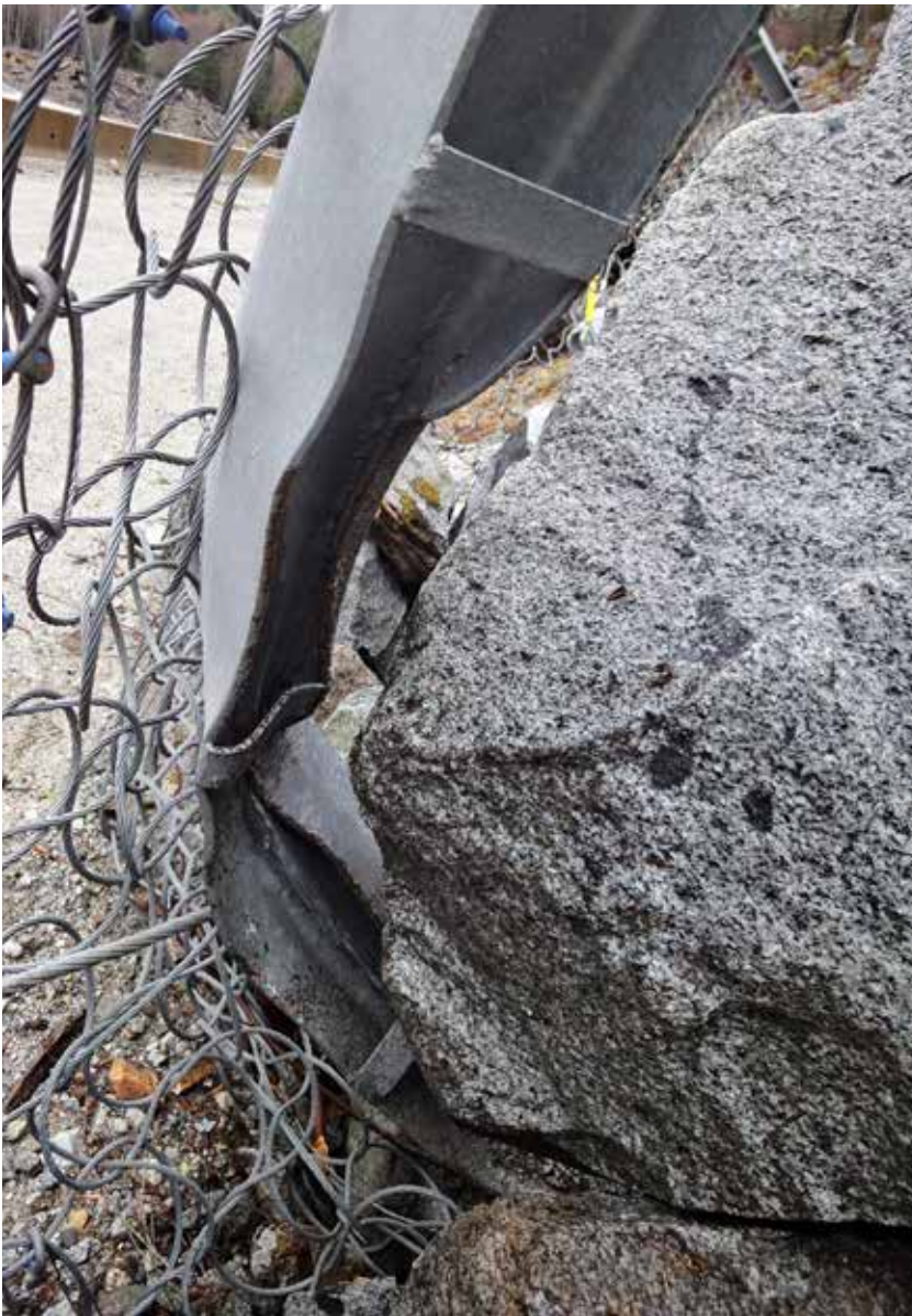
Figure 4. Rockfall barrier post impact in British Columbia, showing continued performance even after impact. (Photo courtesy of Trumer Schutzbauten Canada Ltd.)
