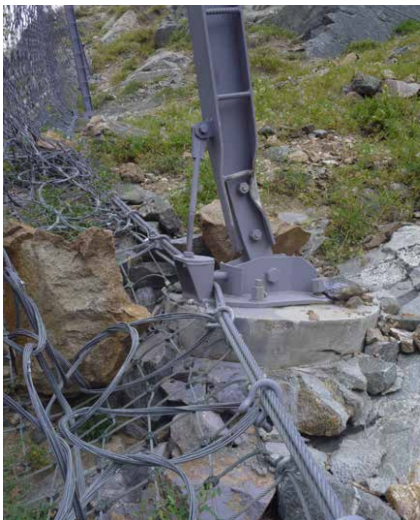
Figure 3. Rockfall barrier post supported on bedrock at Georgetown Canyon, CO, showing continued post-strike performance. (Photo courtesy of Colorado DOT.)
