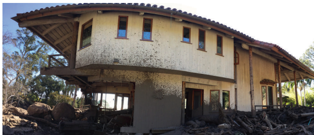
Figure 2. Damaged home along Buena Vista Creek sitting among a debris-flow boulder field and abundant woody debris. Mud line on building is asymmetric, indicating surge-front depths were greater on the left side of the structure (near the top of the handrail on upper floor deck) than on the right side (photo: Brian Swanson, CGS; all photos taken by USGS and CGS unless otherwise noted).
